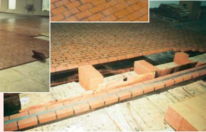
Chemical resistant membrane and brick installation. This proven heavy duty flooring protection system is designed to take rugged treatment and provide maximum resistance to continuously wet chemical conditions.
