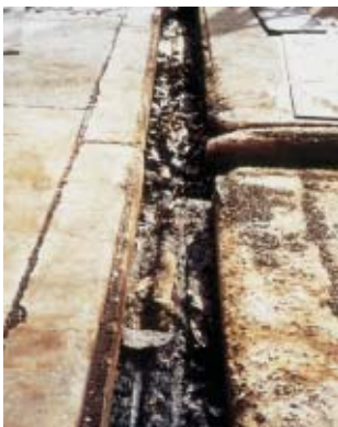
This trench required major refurbishment not only to meet production requirements but also safety and environmental standards
