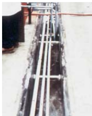
By incorporating an anchored plastic lining with a monolithic topping, the life of this trench was significantly extended at a fraction of new construction costs.
