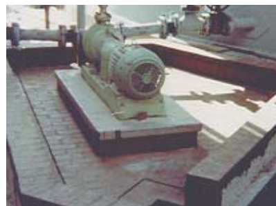
Secondary containment system for extremely harsh acid (37% HCl) utilizes an asphaltic membrane with acid brick and a chemical resistant mortar to protect the underlying concrete.
